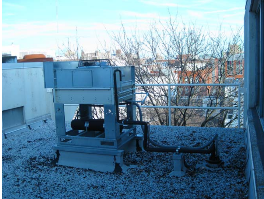
Fig. 1.7. Heat exhaust component of the dedicated chiller for the PPMS system. It is located on the roof directly above the PPMS laboratory.
