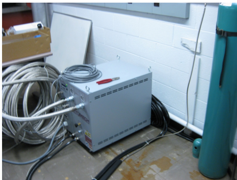
Fig. 1.6. Compressor for the helium recovery and liquification system with black chilled water lines going back to the water chiller system.
