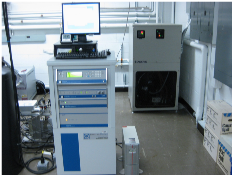
Fig. 1.5. PPMS control system cabinet and computer. To the left on the floor is one of the two UPS systems for the control system. The chilled water reservoir and recirculation system is located in the far right corner.
